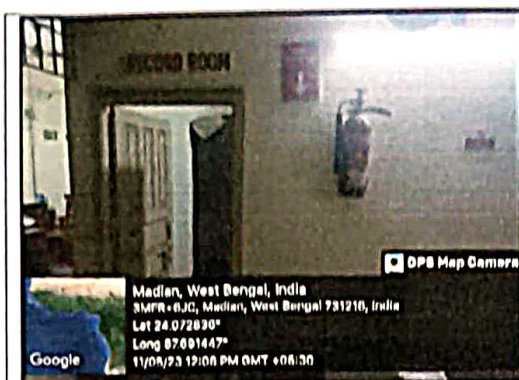
Fire Extinguisher at Record Room Entrance
